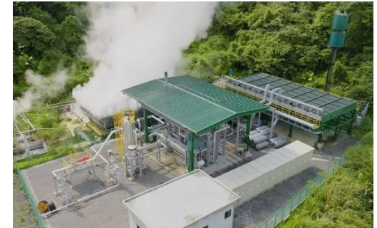
Geothermal ORC Power Plant
